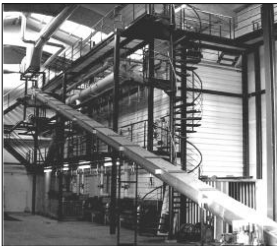
Figure 5: The four vessels of the ROM-sequential batch plant conjoined by a sophisticated piping (located inside a building).
