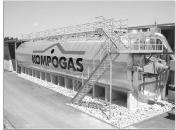
Figure 4: New modular KOMPOGAS-plants are put up outside, enclosing for waste air treatment just the parts producing bad odours.
